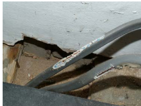
Typical rodent damage in unprotected cable
